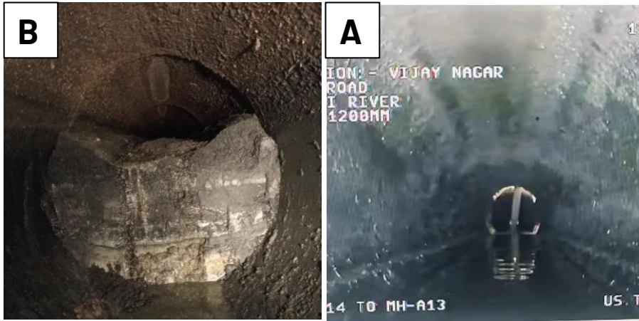
Vijay Nagar North Delhi Trunk Sewer (NTS)
