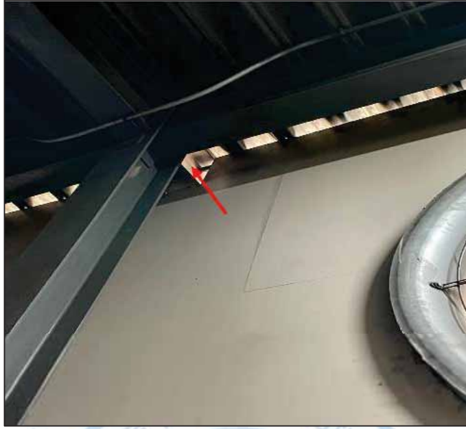
Figure 111. Leak through cut-outs in the pillar.
