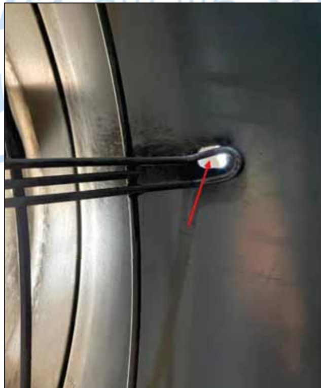
Figure 125. Leak due to the missing bolts of the fans inside the MSACS.
