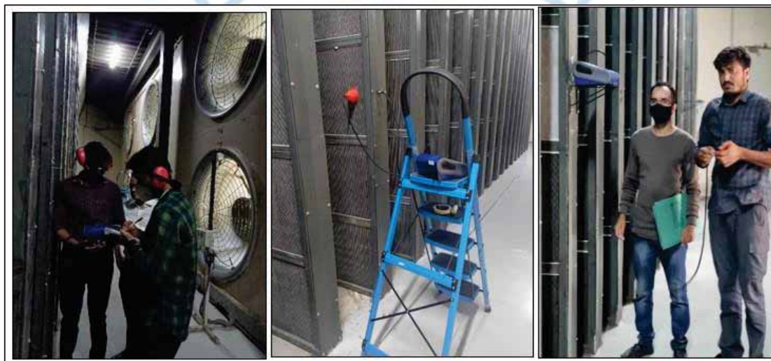
Figure 153. Inside Tower- Filter Measurement.
