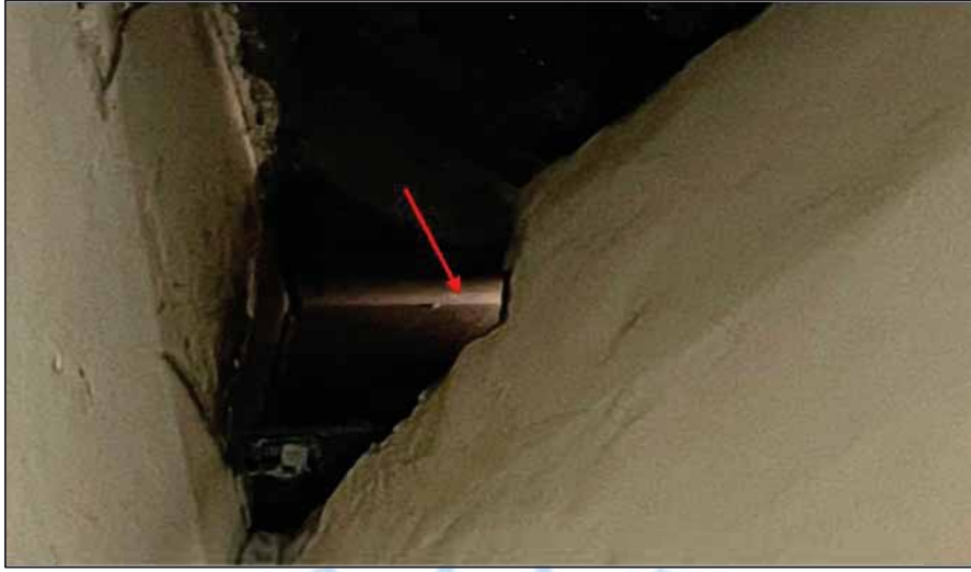
Figure 122. Leak through the openings at the corners inside the MSACS.
