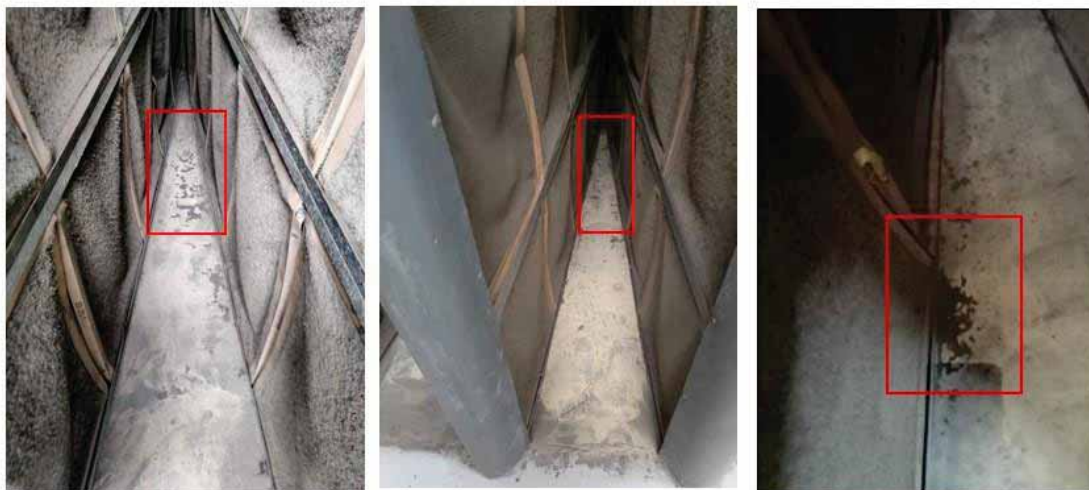
Figure 49. Dust fallen out from the pre-filters on the floor.
