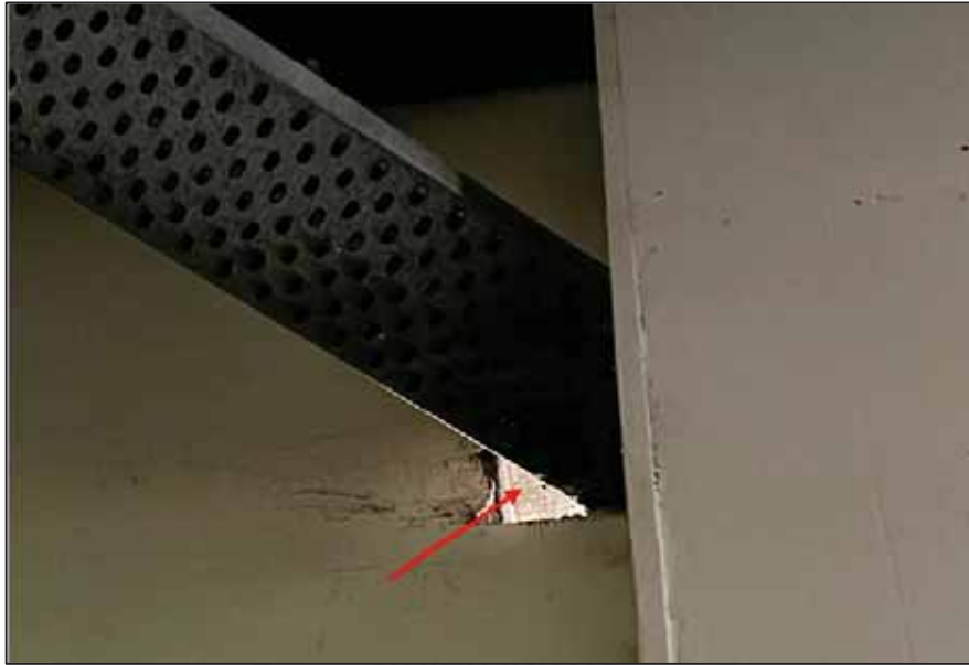
Figure 124. Leak through cut-outs in the walls inside the MSACS.
