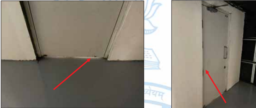
Figure 110. Leak through the opening in the door inside the tower and sometimes when the door remains open.
