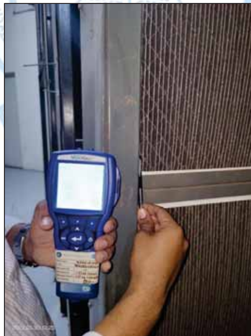
Figure 133. Air coming through gap between filter and filter frame \sim 7.53 m/s.
