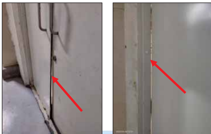
Figure 128. Leak through the main door of the tower.
