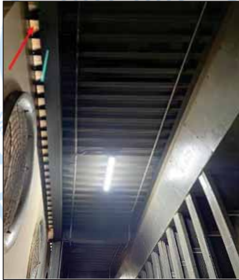
Figure 108. Leak through the cut-outs in the roof and pillar.
