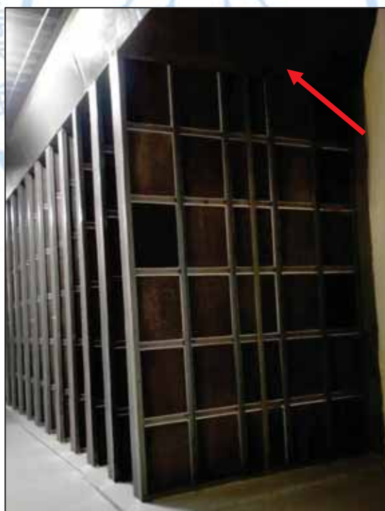
Figure 131. Leak through the top edge of the filter frame.
