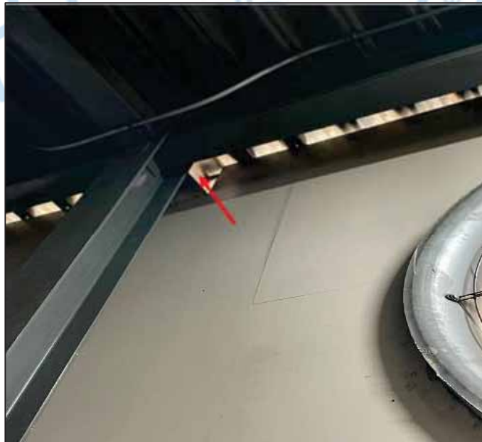
Figure 121. Leak through cut-outs in the pillar.
