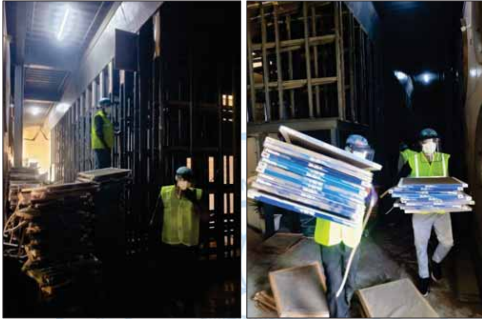
Figure 148. Filter replacement from filter bank.
