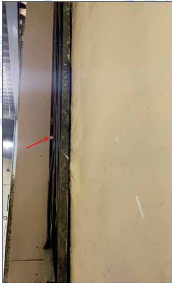
Figure 123. Leak through openings in the pillars inside the MSACS.
