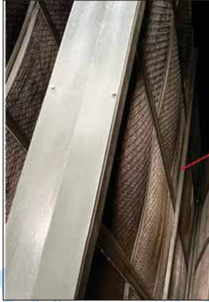
Figure 107. Leak between filters due to the distorted edge.
