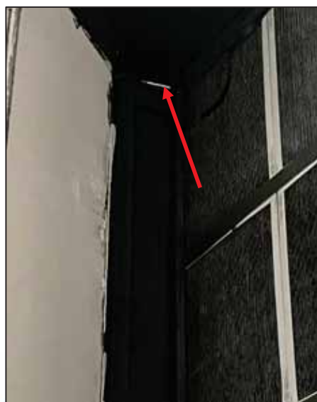
Figure 113. Leak through cut-outs near the walls inside the tower.
