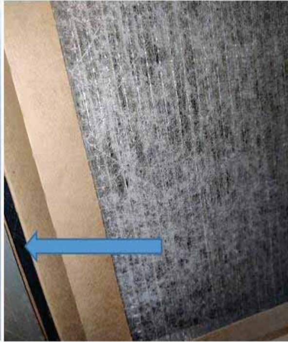
Figure 11. Gaps spotted between the pre-filters.
