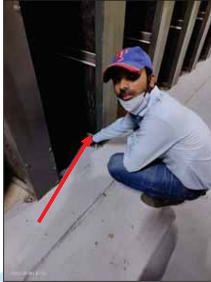
Figure 126. Leak through the bottom edge of the filter frame.
