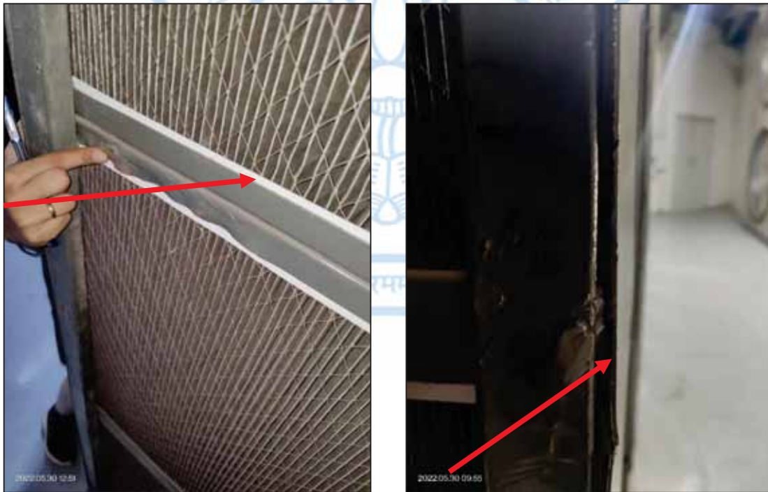
Figure 127. Leak between filters due to edge gaps and gap at end plate.
