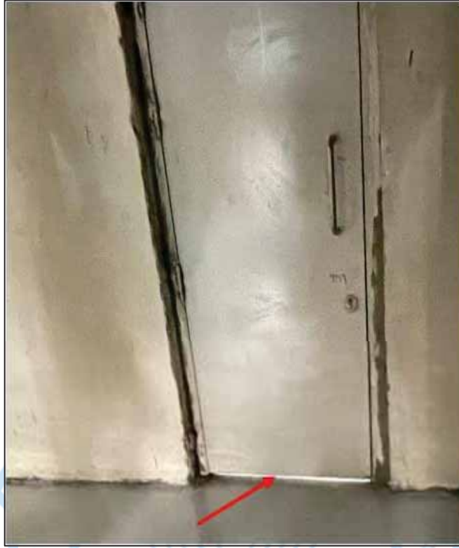
Figure 120. Leak through the opening in the door inside the MSACS.
