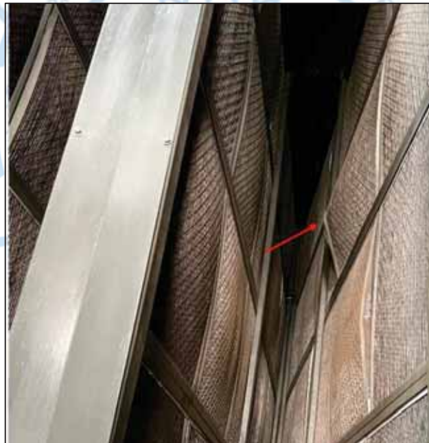
Figure 117. Leak between filters due to distorted edge.
