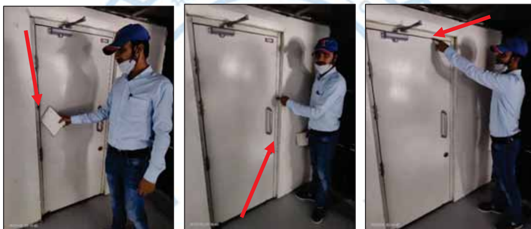
Figure 129. Leak through the opening in the door inside the tower. ( Upstream opening to internal door is requested )
