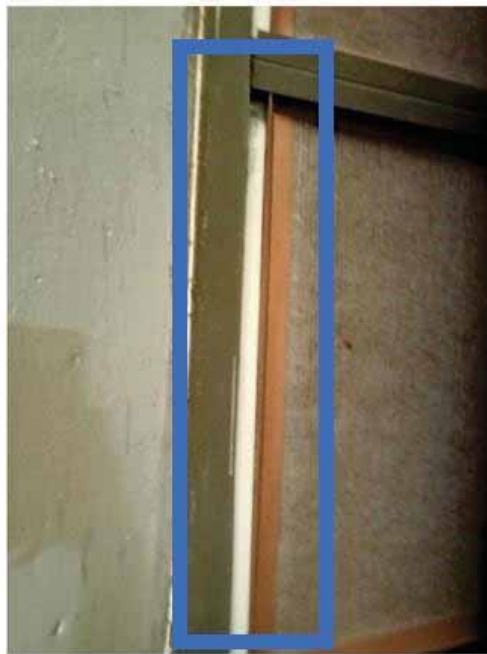
Figure 12. Gaps created between the pre-filters and filter frame.
