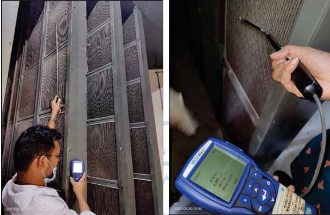
Figure 132. Actual air coming through filter \sim 0.27 m/s.
