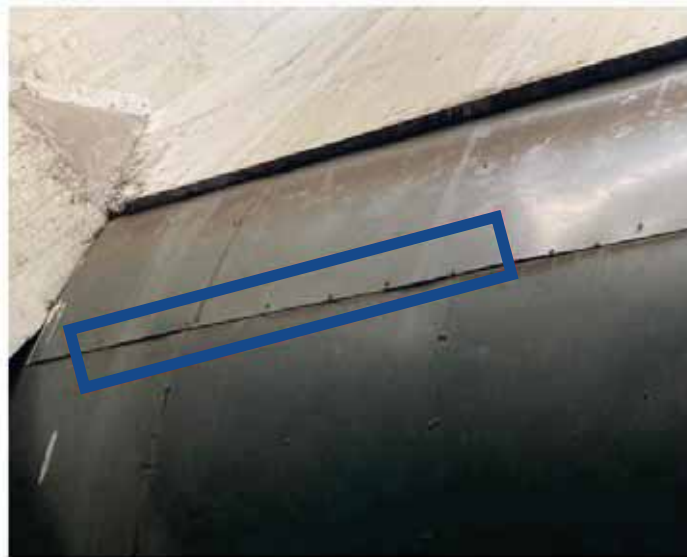
Figure 14. Leaks in the structural joints.
