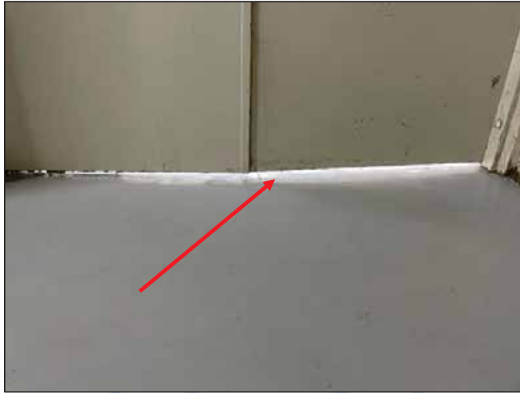
Figure 109. Leak through the main door of the tower.
