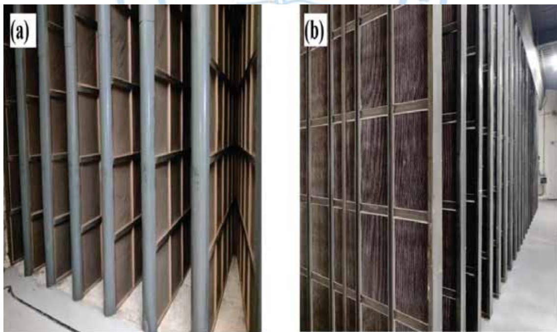
Figure 19. Visual observations on the condition of filters in November 2022 (a) Pre-filters and (b) Fine filters.
