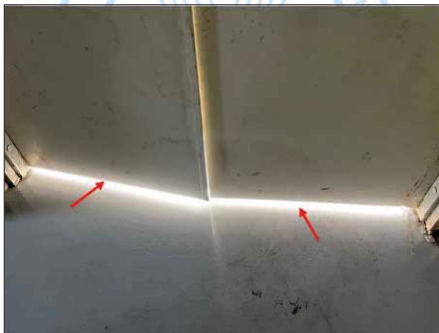
Figure 119. Leak through the main door of the MSACS.
